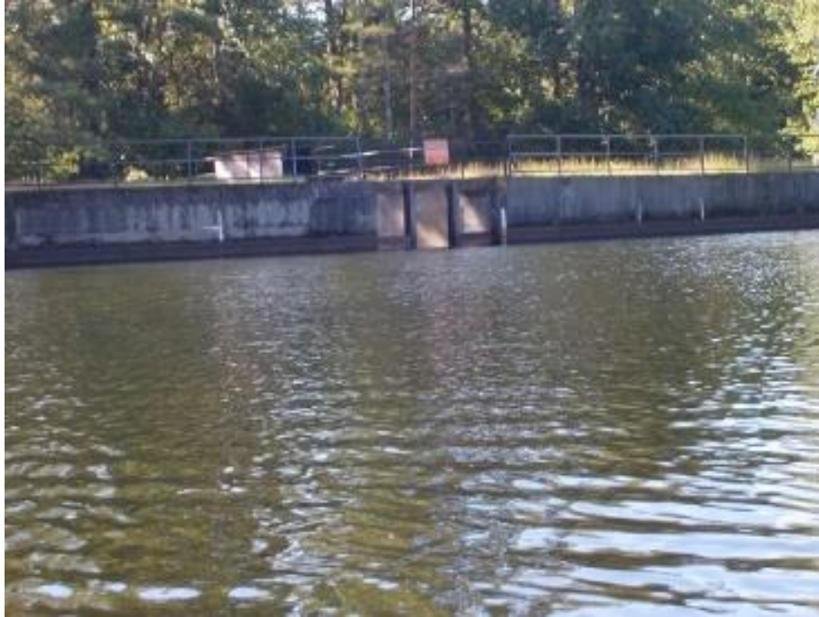
Dolloff Dam with middle two stop logs removed 9 AM August 31, 2022.
