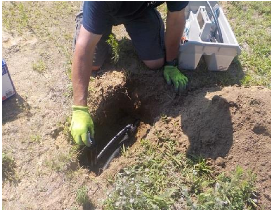
Sprinkler left, connecting piece middle, the buried hose right
