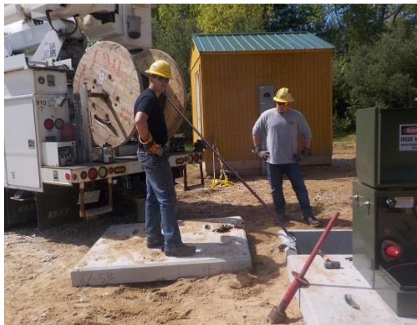
Of NHEC, left Colin McDonough and right Randy Cosborne with the high voltage cable being plied out to the powerlines with the transformer on the right.
