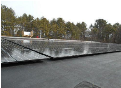
Solar Panels installed on Nottingham's Community Center roof 2018
